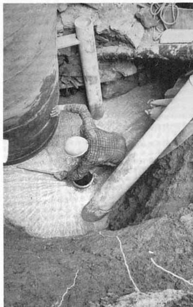
Concrete slab over the rift, and water pipes from the settling tank.
