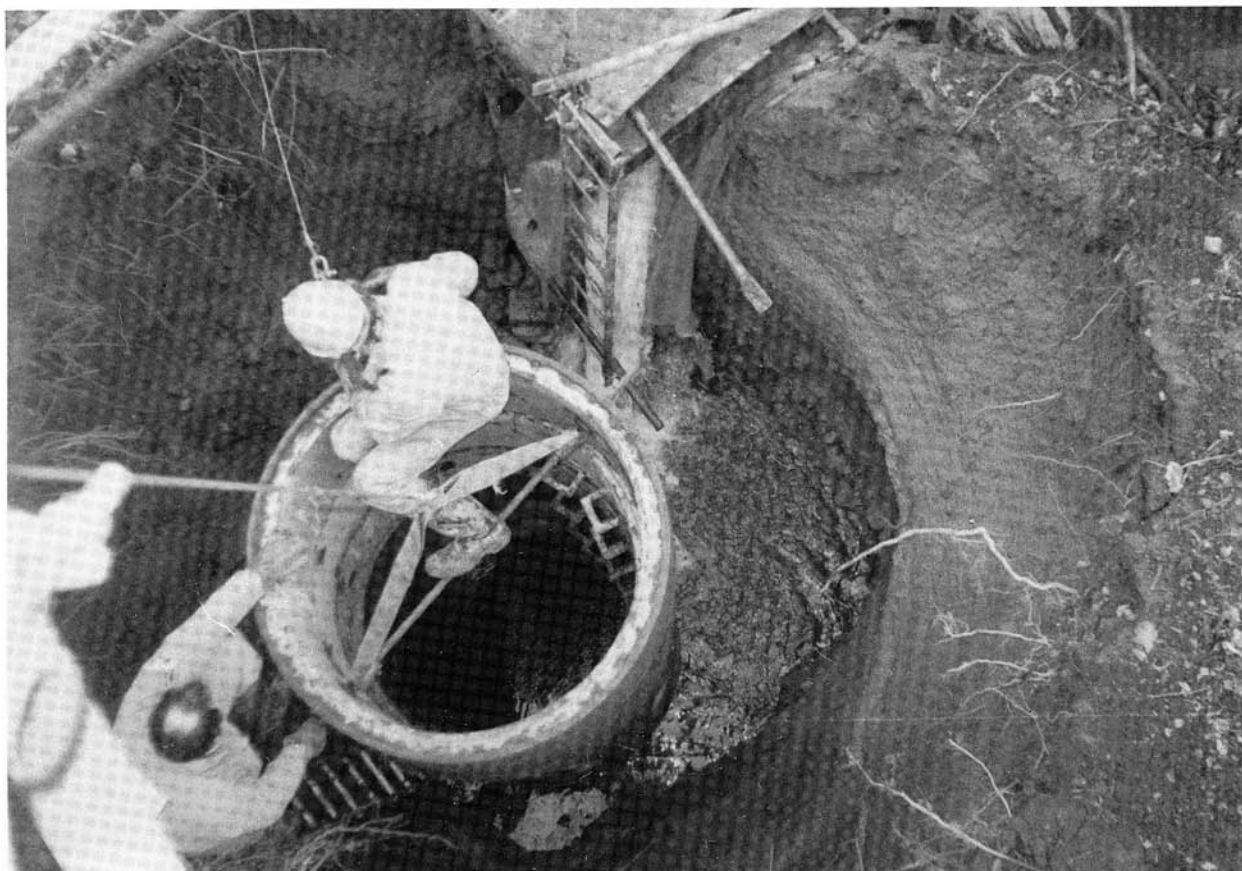
The last ring goes onto the stack; this photograph was taken from on the jib above the hole.
